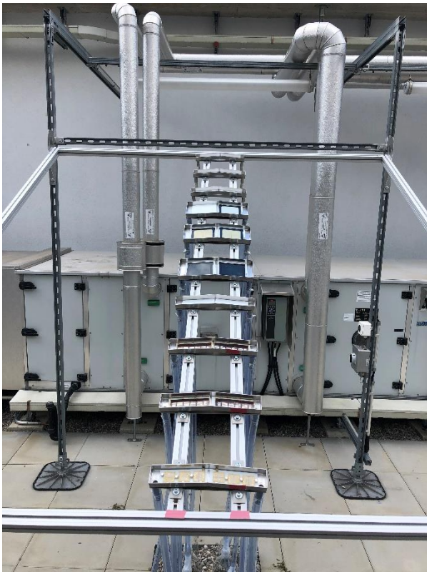
Figure 11: Image of constructed outdoor installation. Stainless steel mounts were constructed to place the PSCs and include a drain for the collection of rainwater.
